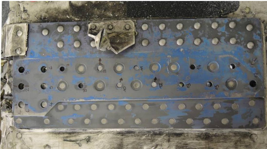
Figure 59: The flexible plate aft attachment had detached from the fuselage plate. 9 out of 17 bolts were still in place. Arrows indicating direction of overload in shear (towards the left relevant to the helicopter direction of flight). Photo: AIBN
