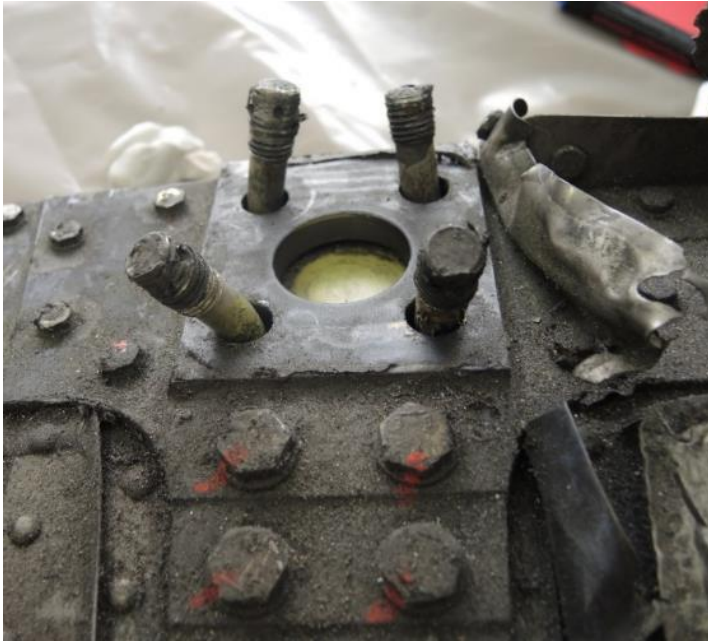
Figure 58: The four bolts from the lower forward fuselage fitting protruding from the support plate. Photo: AIBN
