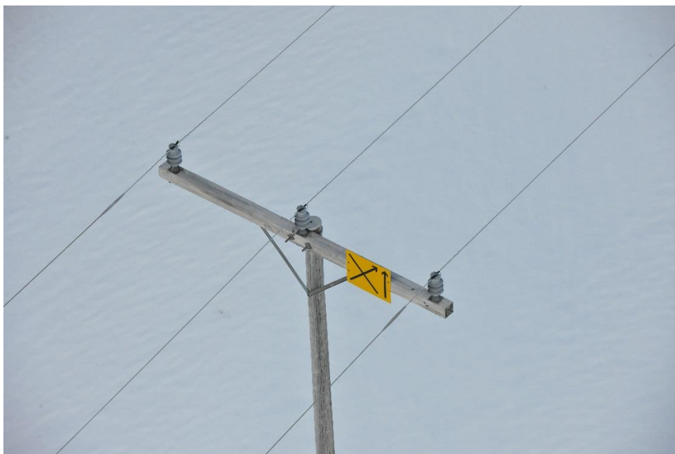
Figure 6: Signs on Helgeland Kraft's power distribution network notifying of an upcoming crossing line ahead. Photo: Pegasus AS
