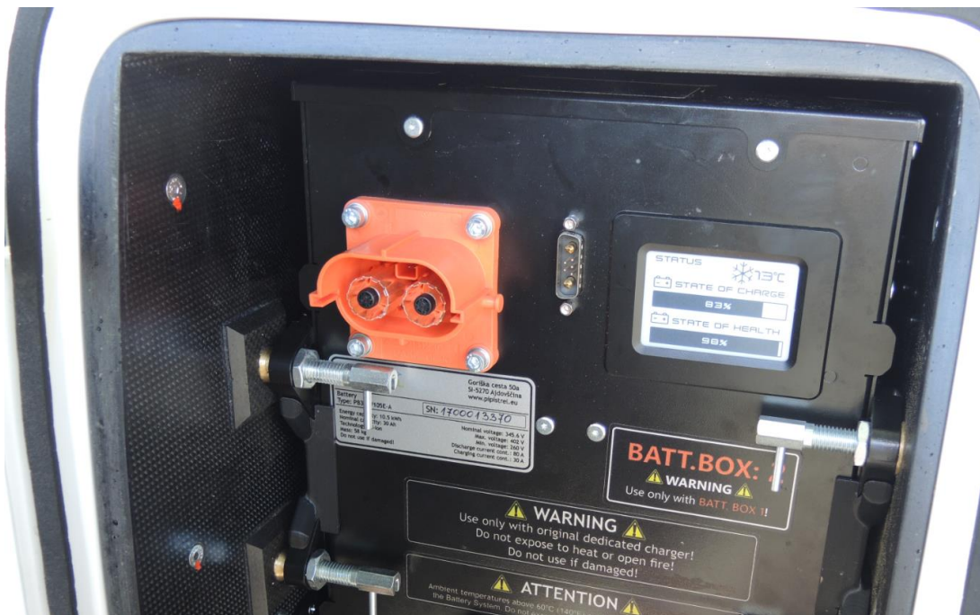
Figure 16: The charge status of the aft battery box was 83%, and the battery state of health was 93%. Photo: NSIA
