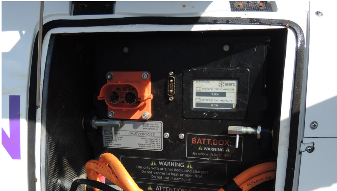
Figure 15: The charge status of the forward battery box was 78%, and the battery state of health was 97%. These readings were taken after the battery box had been submerged in water. Photo: NSIA
