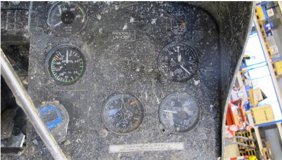
Figure 8: The artificial horizon should have been installed under the sign “Radiocall LN-OBP”. The hole after the instrument was covered with electrical tape. Photo: NSIA
