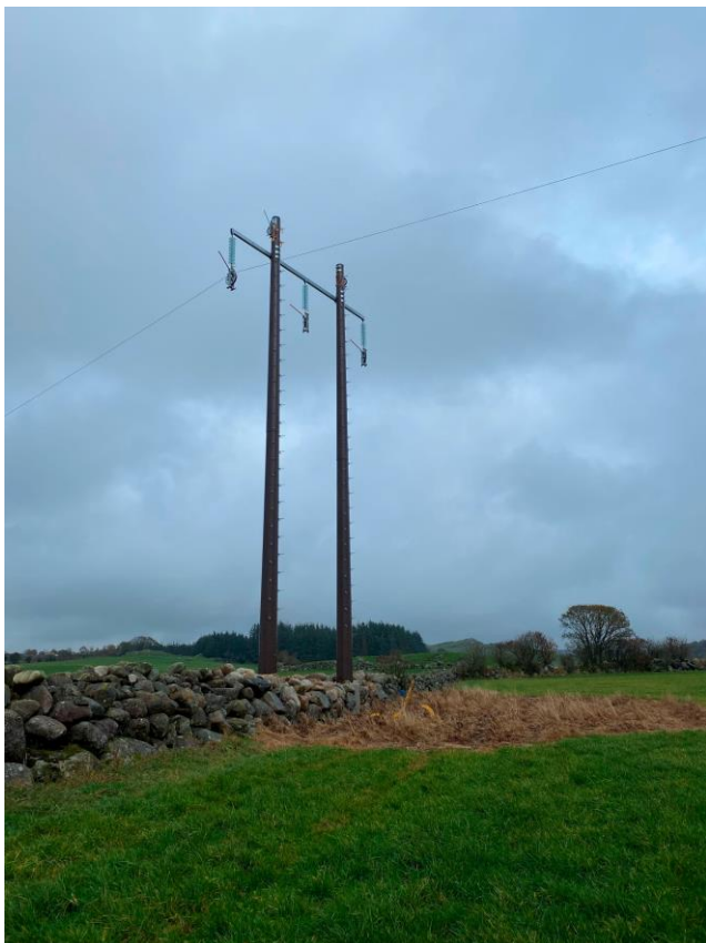
Figure 2: The actual mast where the incident happened. Photo: Helitrans/NSIA
