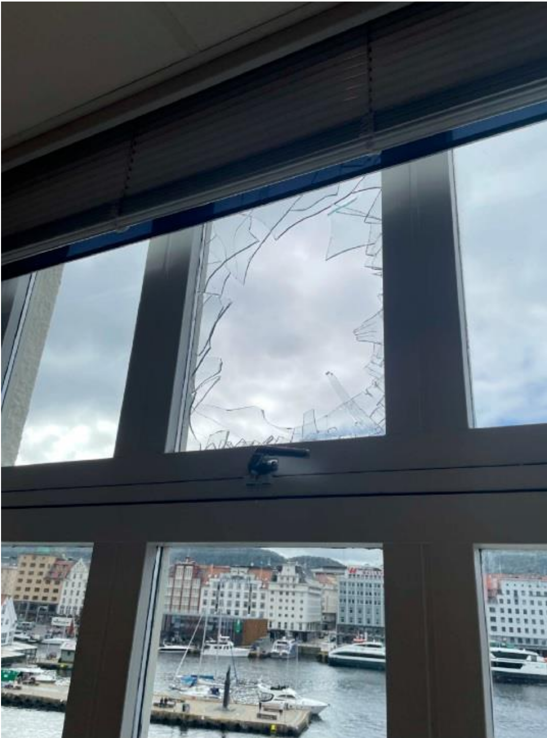
Figure 9: Damage to the window the drone crashed through. Source: Police / NSIA
