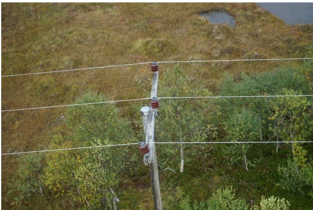
Figure 4: An example of a crossarm with damage inspected the same day as a part of the power line inspection. Photo: Vesterålskraft Nett AS / NSIA
