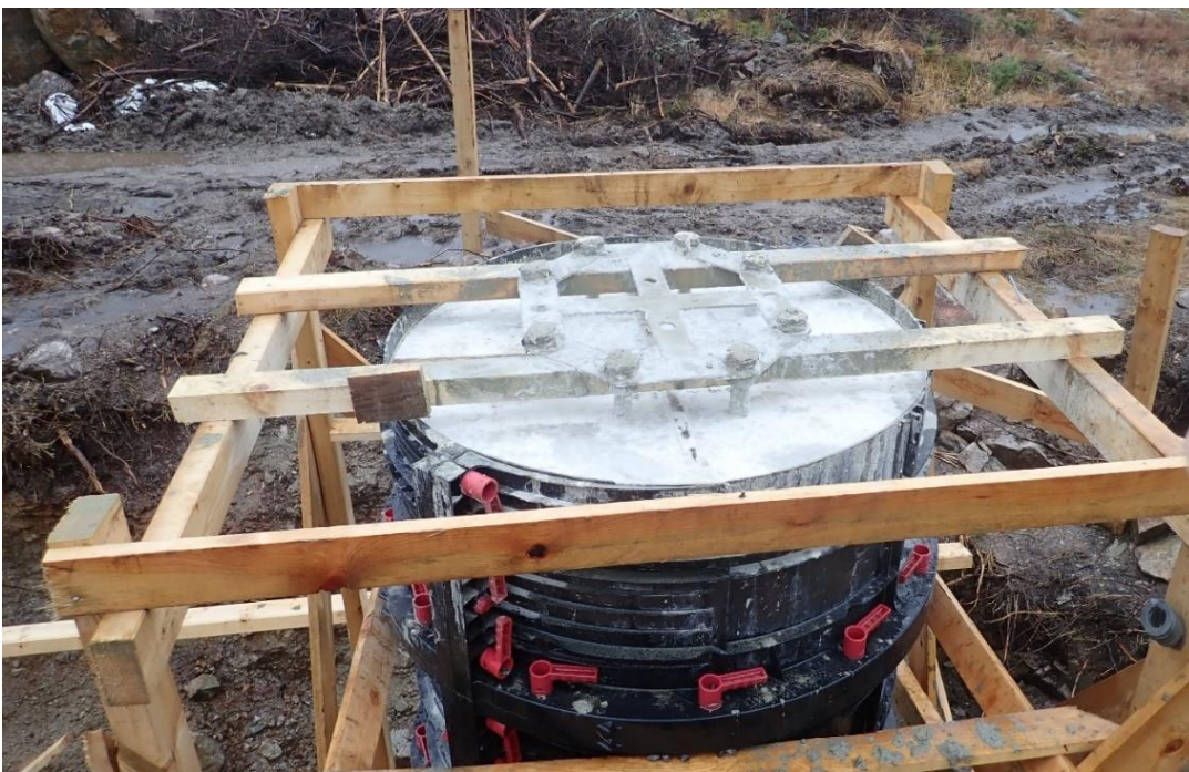
Figure 2: Pylon foundation 49, the day after the accident. Casting of the foundation had then been completed. Photo: NSIA
