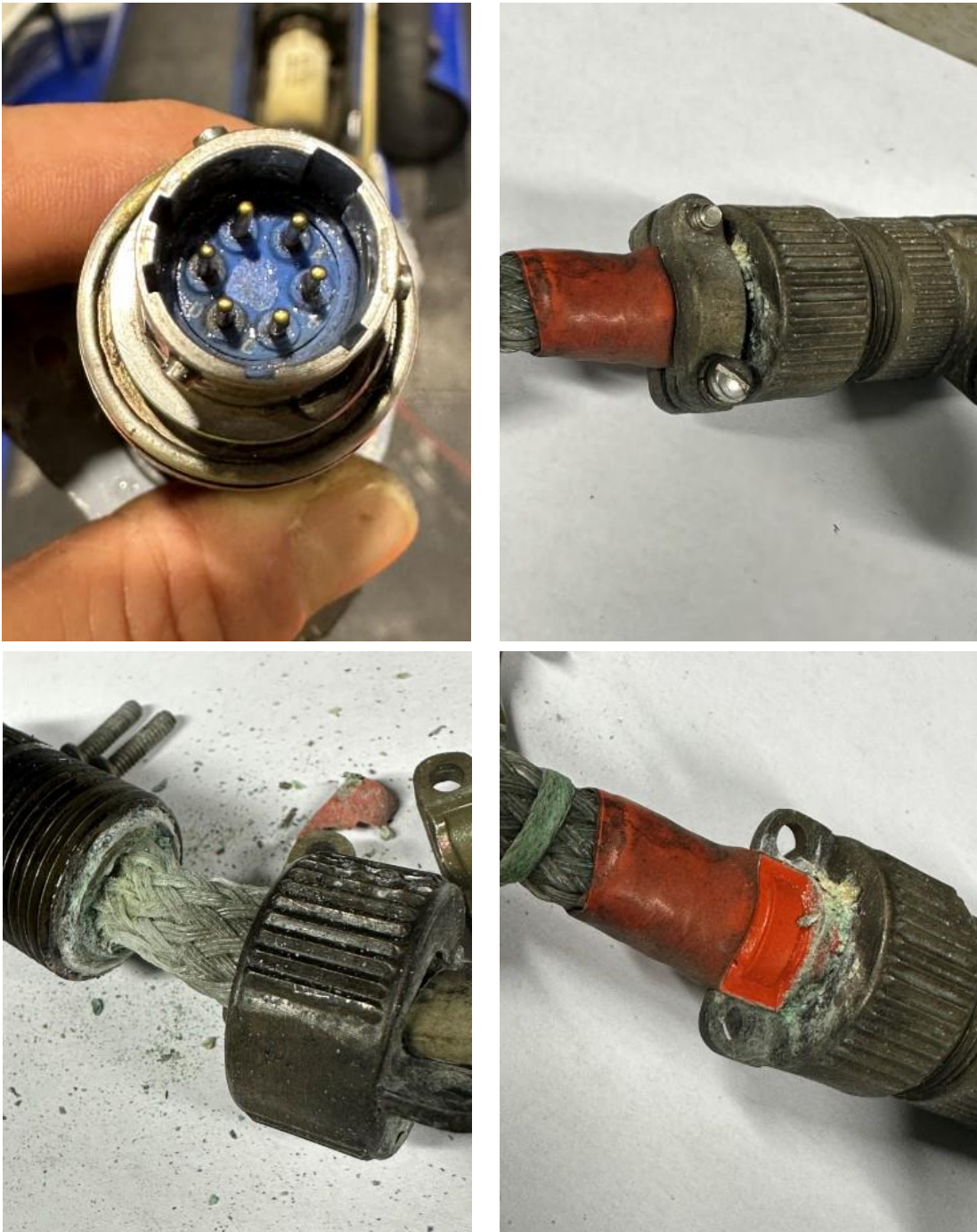
Figure 5: Examples of corrosion found on connectors in the S-92's fire warning system at Bristow's facilities. Photo: Bristow Norway/NSIA
