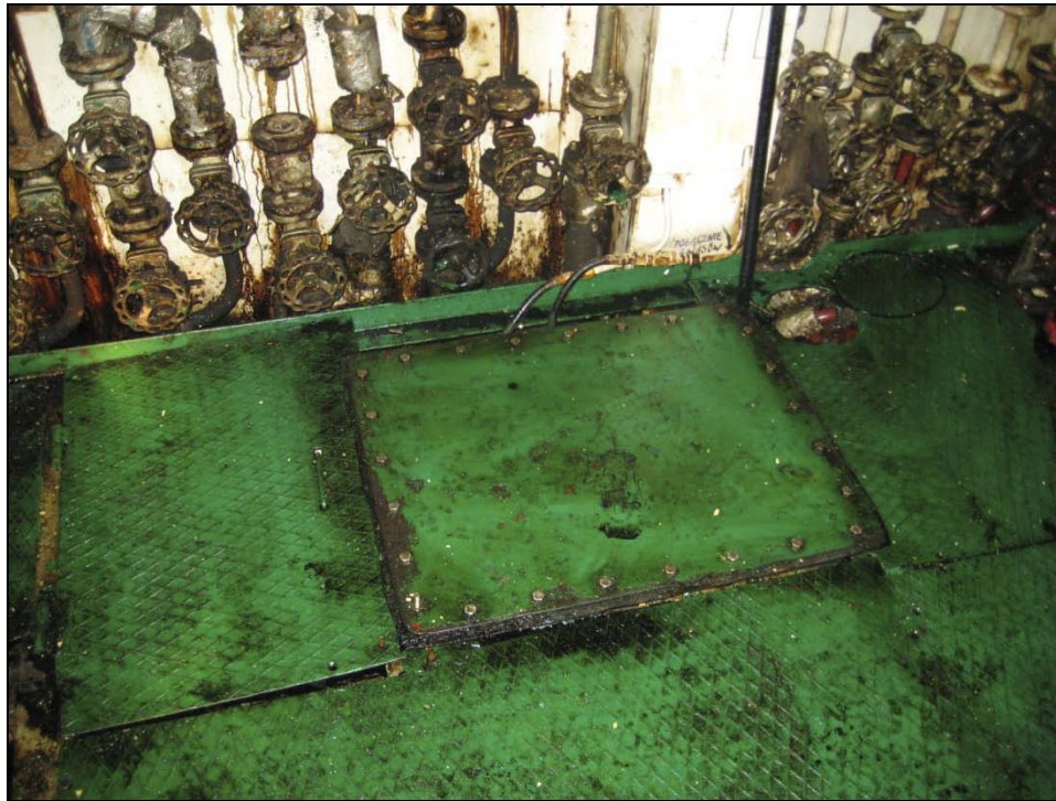
Figure 17: Manhole cover in engine room for access to the pipe trunk.
