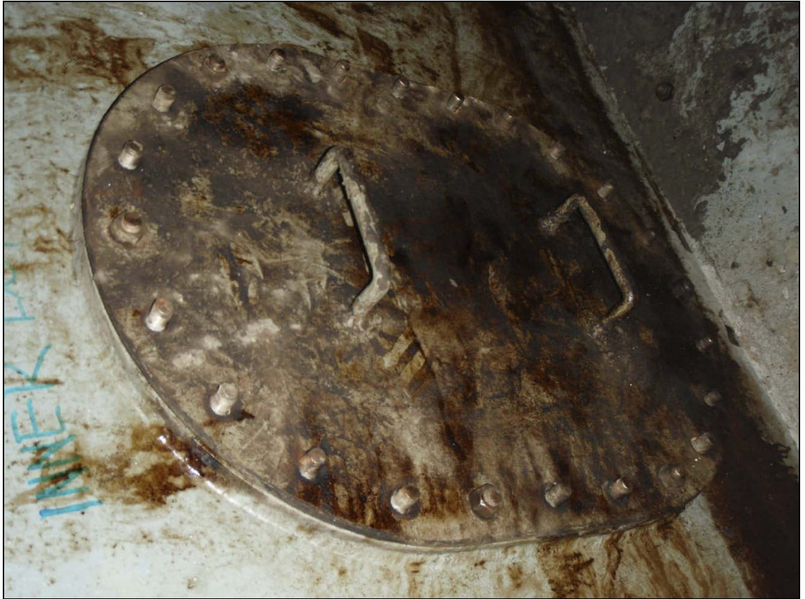
Figure 4: Manhole cover from the blow-tank tunnel towards the void below the cargo hold.
