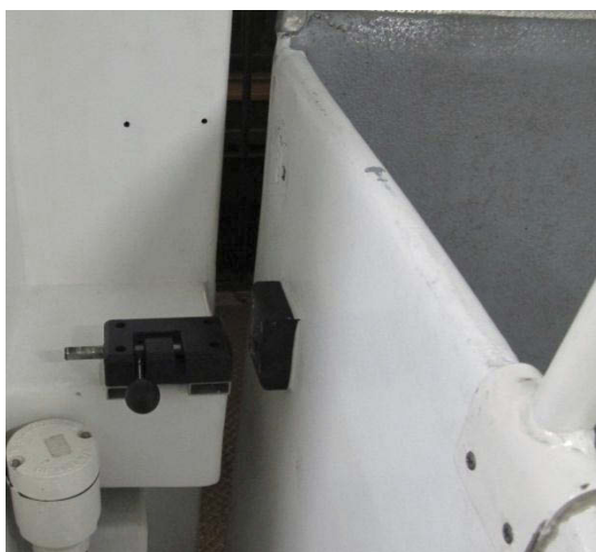
Figure 6: The locking bolt for the starboard gangway on the aft deck is not secured. Photo: AIBN.
