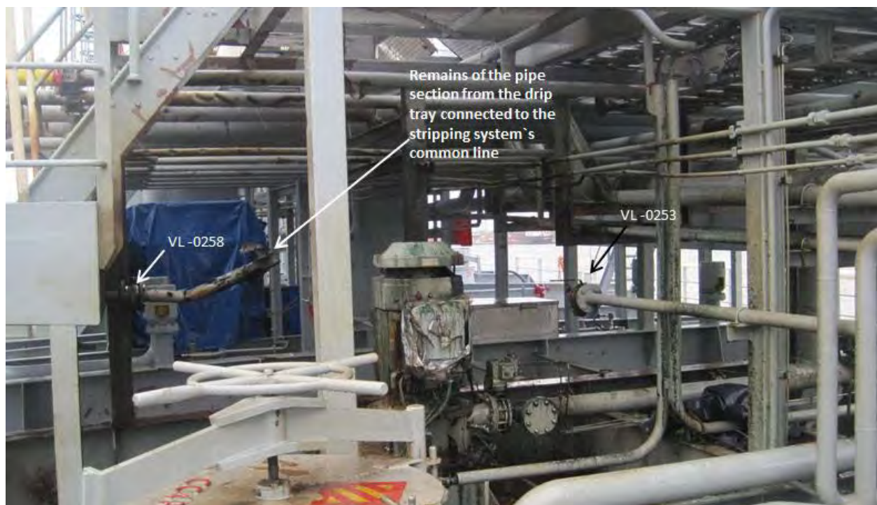
Figure 21: The figure shows the remains of the pipe section from the drip tray on the port side to the drainline after the explosion, cf. Figure 20. Photo: AIBN
