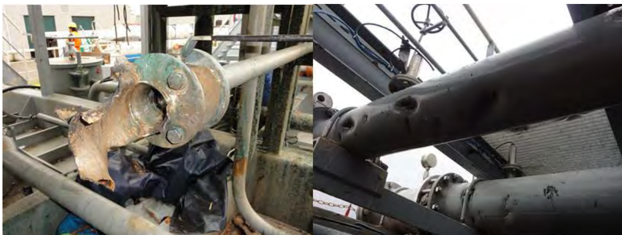
Figure 8: The photo on the left shows the drainline that was blown up. The photo on the right shows one of the cargo lines perforated by flying parts of the drainline. Photo: Capt. Hugo Vereckeen
