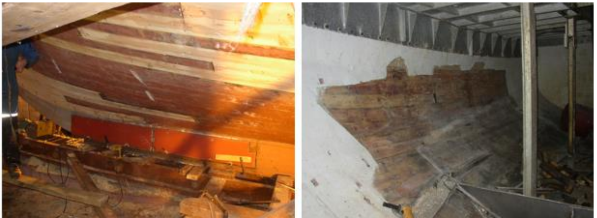
Figure 10: The photo on the left shows some of the replaced shell planks. The photo on the right shows the cargo hold with the bottom removed. Photo: Grovfjord Båtbyggeri AS
