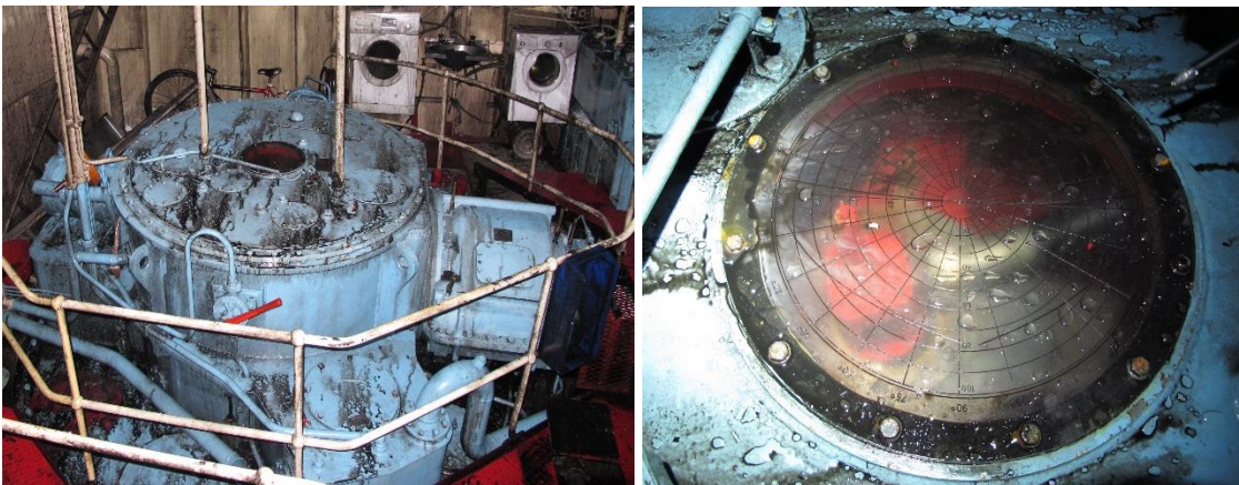
Figure 25: Starboard propeller unit. Photo: AIBN
