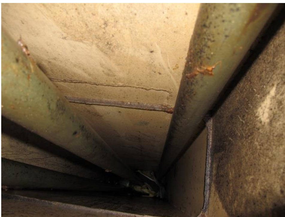
Figure 18: The three pitch rods passing vertically through the trunk to the engine room. Photo: AIBN
