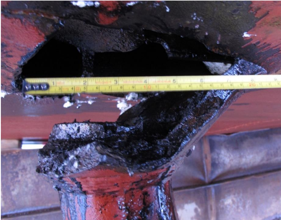
Figure 5: The rear inner strut on the starboard side had torn open the skin of the hull. Photo: AIBN
