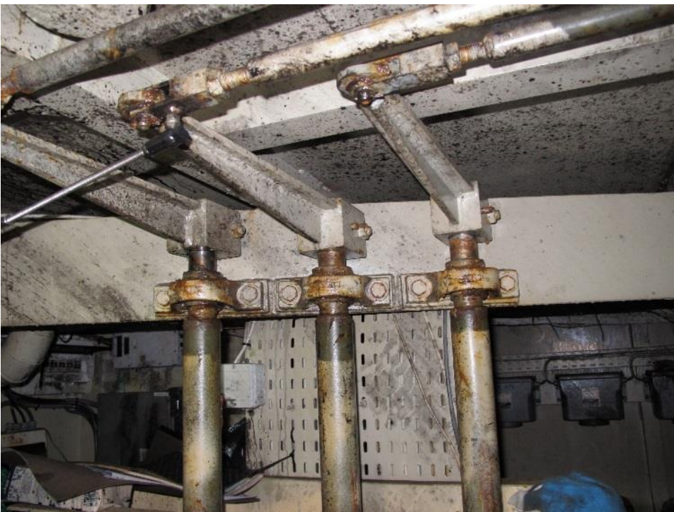
Figure 16: Longitudinal movement transfer via the three horizontal rods to rotation in vertical rods. Rudder pitch in the middle. Photo: AIBN
