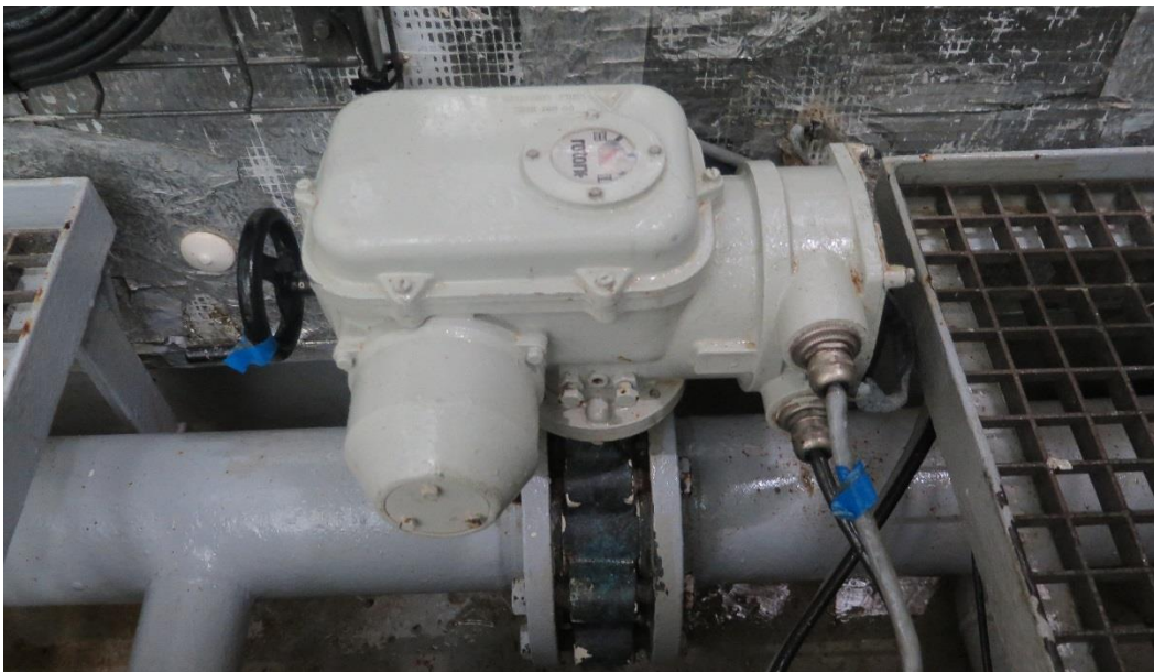
Figure 74: Example of isolation valve. Photo: NSIA
