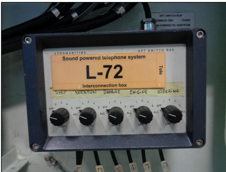
Figure 48: Conference box for SPT. Photo: NSIA
