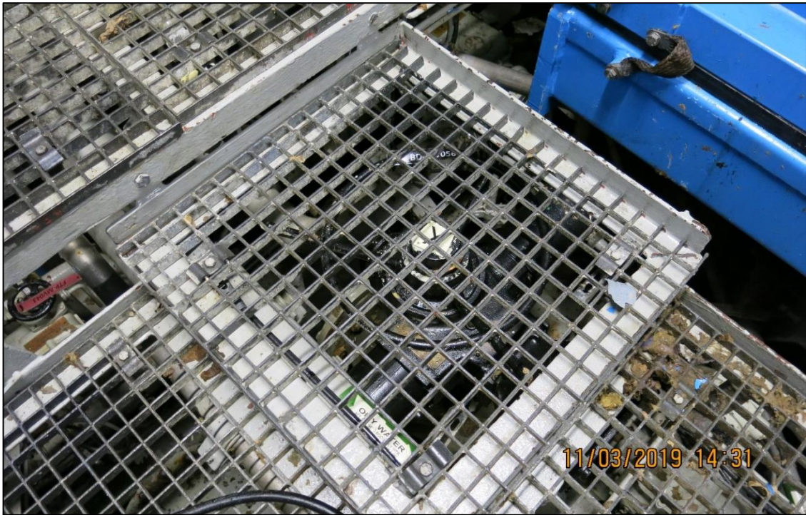
Figure 57: Suction valve (tag BD-MV056) in black, located under floor grate in the aft generator sets room. Photo: NSIA
