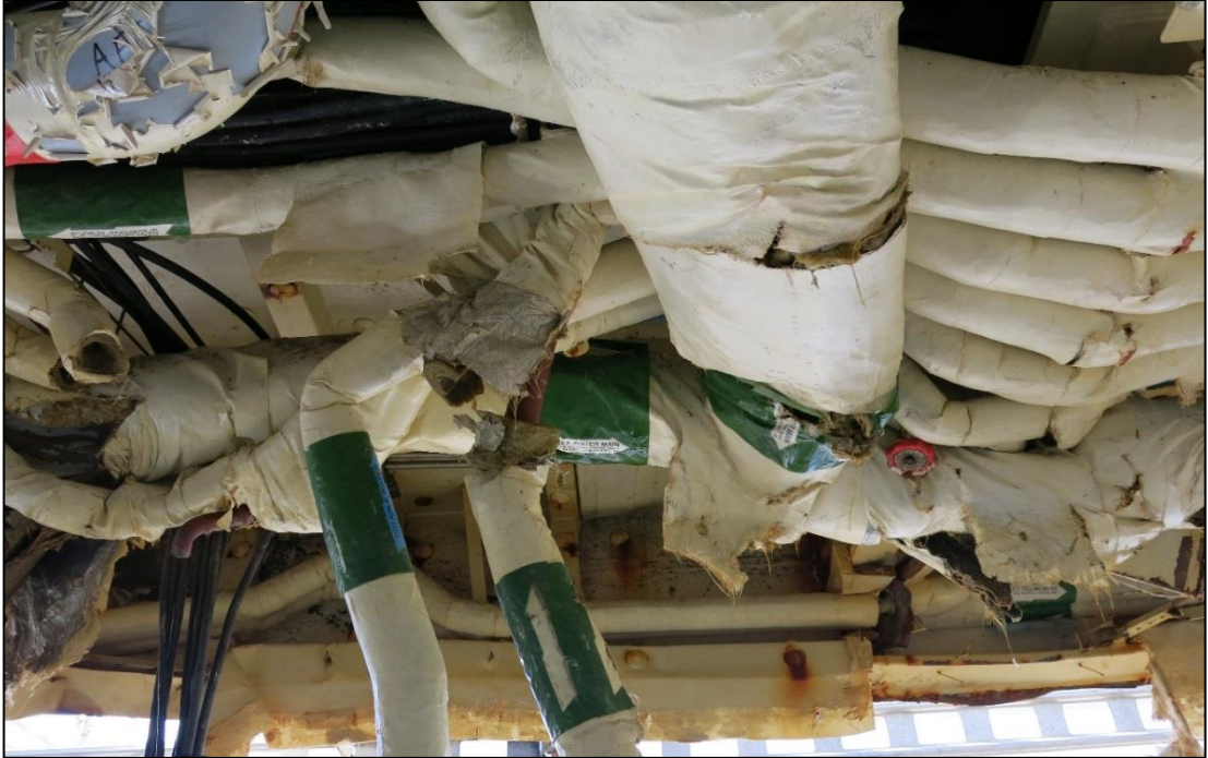
Figure 22: Damage to the seawater main aft of fire zone 4. Photo: NSIA
