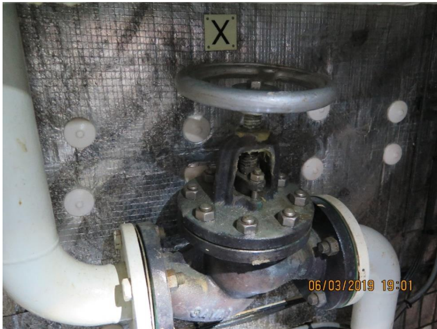
Figure 73: Example of manual bilge valve marked with an 'X' in the bilge system. Photo: NSIA
