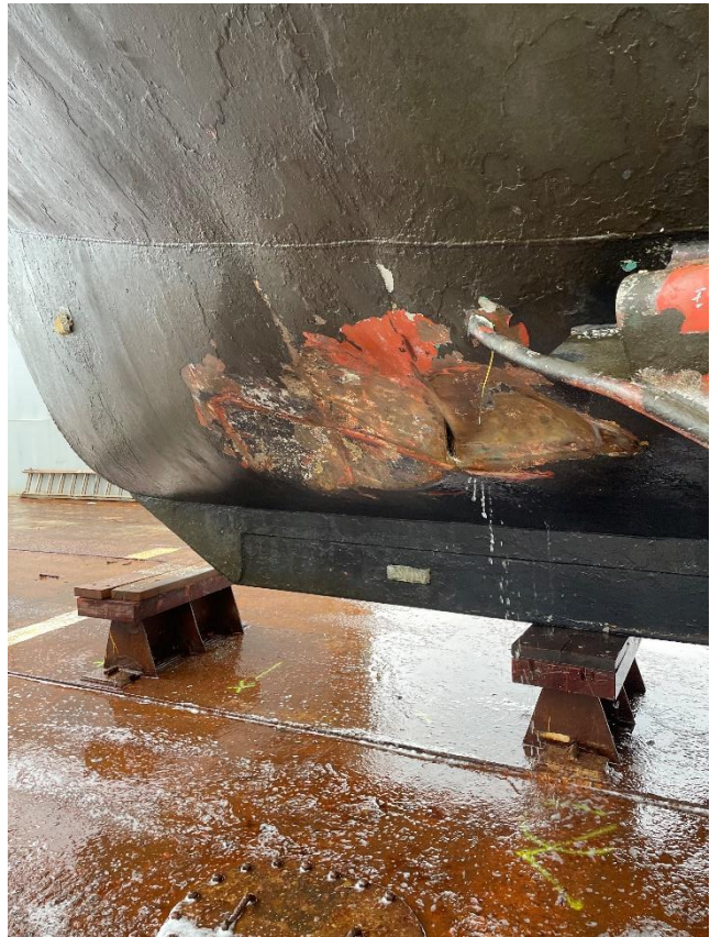
Figure 7: Damage to the hull that resulted in ingress of water into the cargo hold. Photo: NSIA
