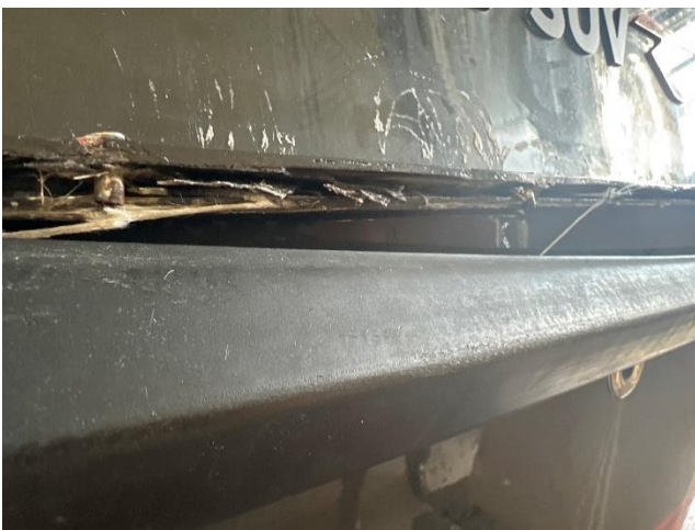
Figure 3: Pop rivets out of position, view from the rear. Photo: NSIA
