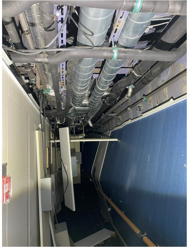
Figure 37: Damage to corridor and ceiling. Forward view. Photo: NSIA
