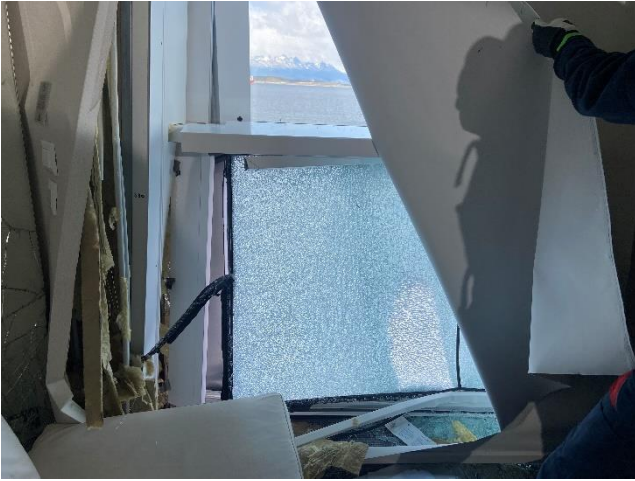
Figure 19: Damage to window and frame in stateroom 2008. Photo: NSIA
