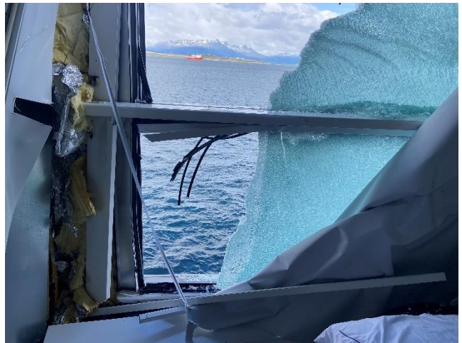
Figure 22: Damage to window and frame in stateroom 2010. Photo: NSIA
