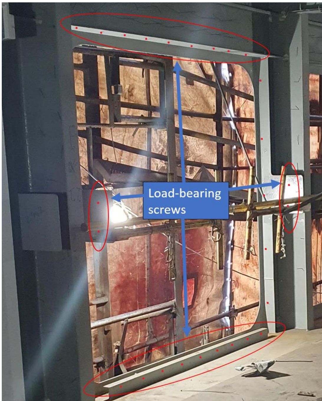
Figure 73: Screws fastening. The red dots show the location of the screws. The load-bearing screws are highlighted. Photo: Window supplier / modified by the consultant
