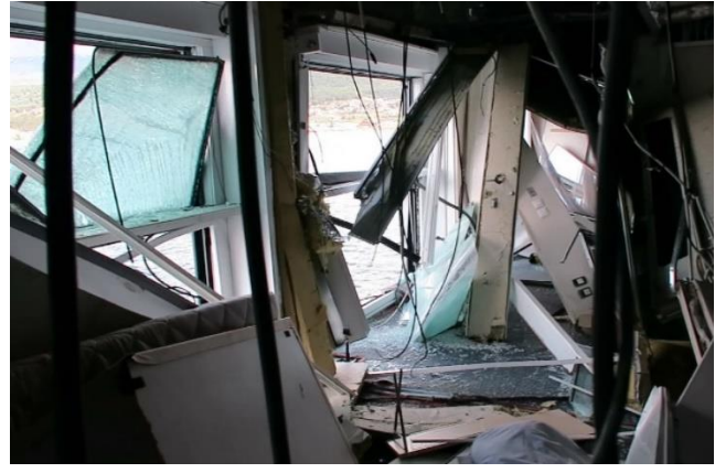
Figure 14: Broken windows in staterooms 2016 and 2014. Photo: NSIA
