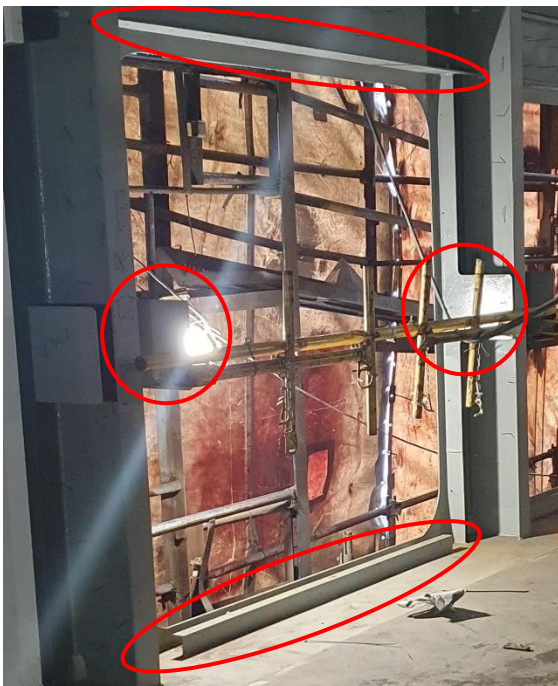
Figure 61: Photo: The window frame was fastened with bolts on the top and bottom. The stiffener was fastened to the plates on either side; as indicated by the red circles. Photo: Shipyard / modified by NSIA
