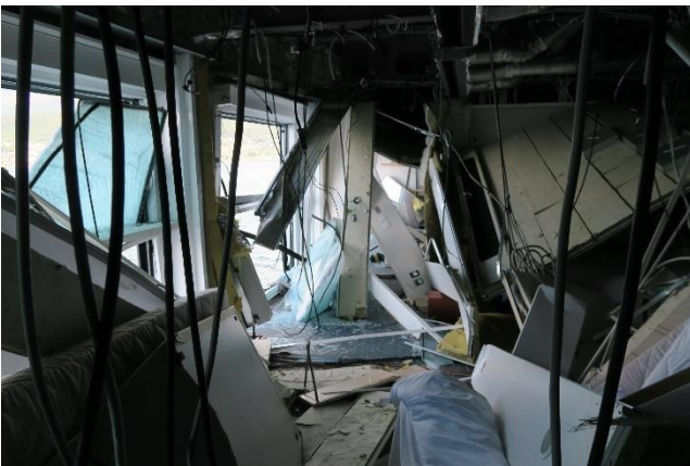
Figure 34: Photo taken from stateroom 2018 also showing damage to staterooms 2016, 2014 and 2012. Photo: NSIA
