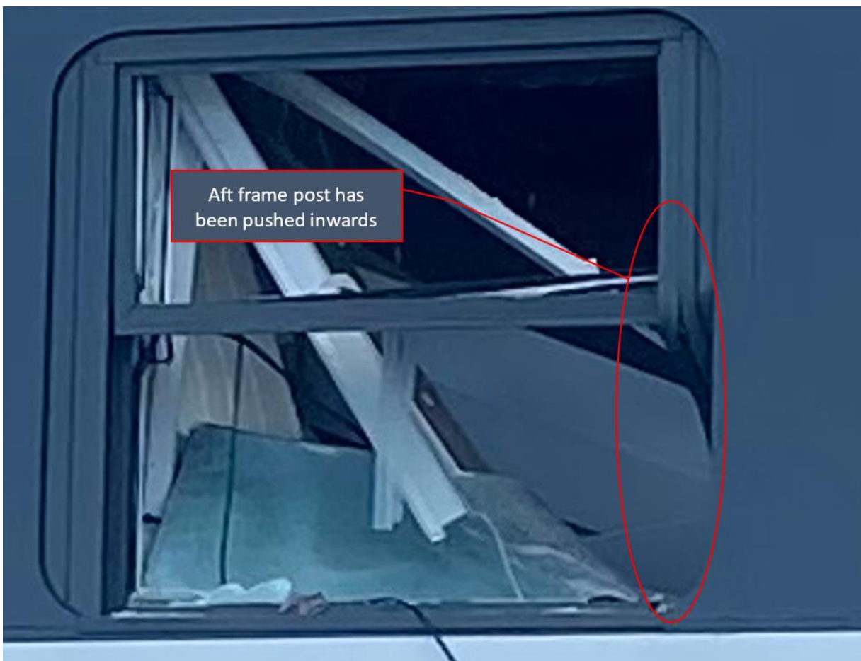
Figure 75: Frame post pushed into stateroom 2014. Photo: NSIA/consultant
