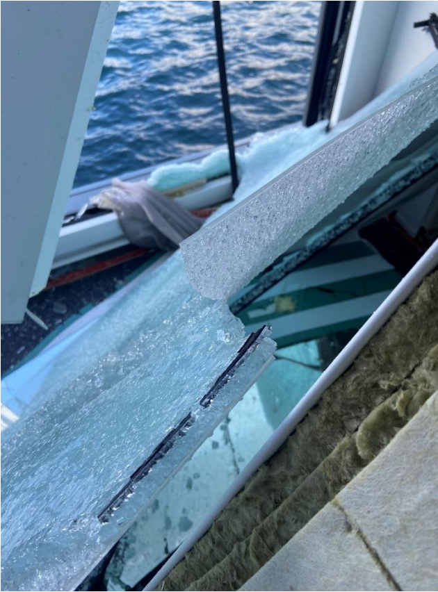
Figure 24: Damage to window in stateroom 2014. Photo: NSIA
