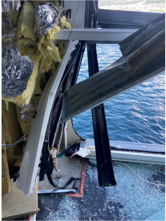
Figure 25: Damaged window frame in stateroom 2014. Photo: NSIA
