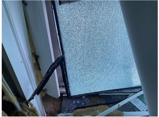
Figure 20: Damage to window and frame in stateroom 2008. Photo: NSIA
