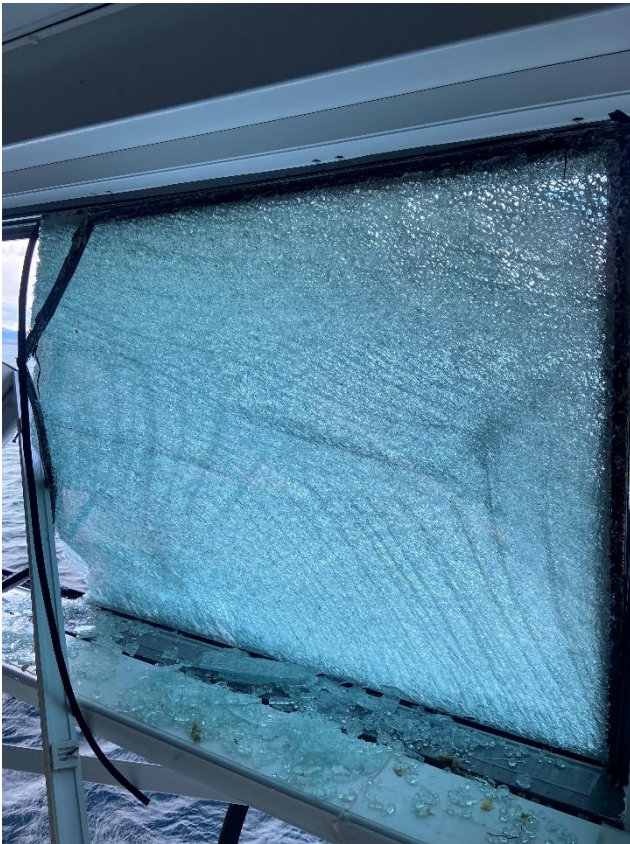
Figure 26: Broken window in stateroom 2016. Photo: NSIA
