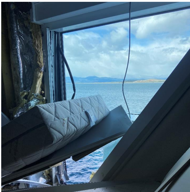
Figure 30: Damage to window and frame in stateroom 2020. Photo: NSIA
