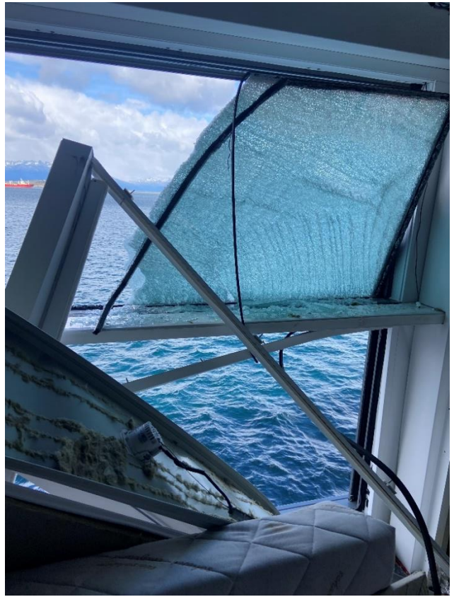
Figure 27: Broken window in stateroom 2016. Photo: NSIA
