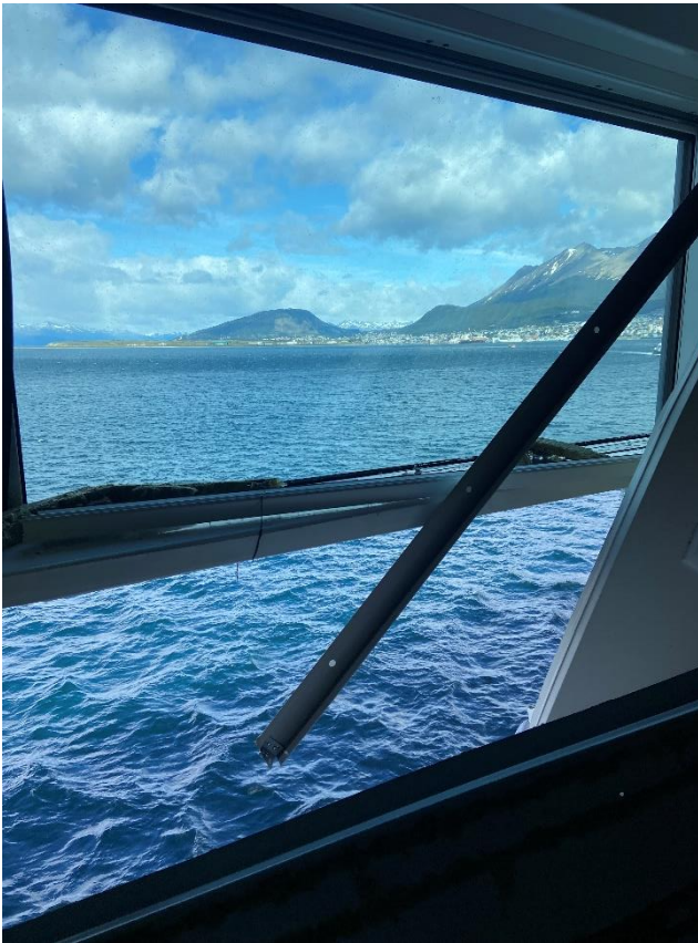
Figure 28: Damage to window in stateroom 2018. Photo: NSIA
