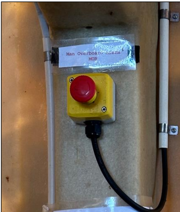
Figure 12: MOB alarm. Photo: NSIA
