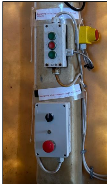
Figure 13: Emergency stop button, conveyor belt. Photo: NSIA
