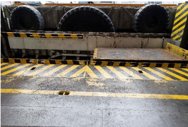
Figure 7: The aft cargo lift was stationary and flush with the upper cargo deck at the time of the accident. Photo: The police
