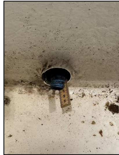
Figure 16: Penetration from the drain in the wheelhouse and into the hold. Photo: NSIA
