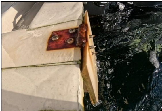
Figure 25: Port drain opening in closed position. Photo: NSIA
