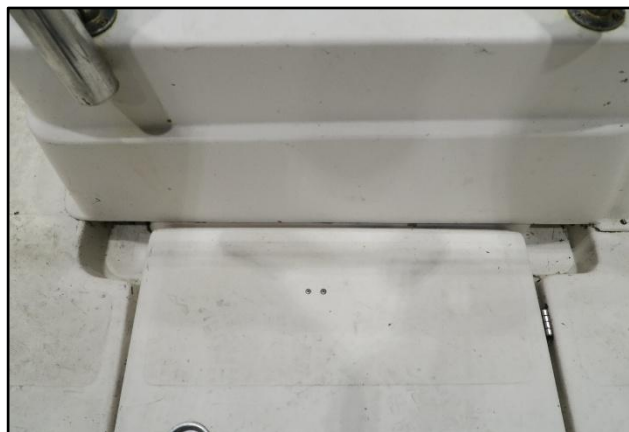
Figure 14: Drainage channels that lead the water out through the drain openings. Photo: NSIA
