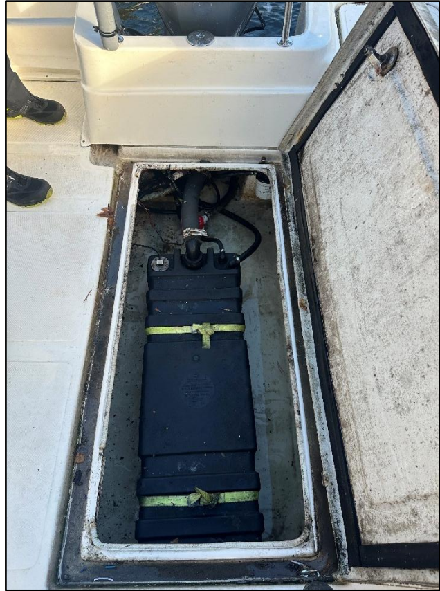
Figure 24: New hatch seal in the flush hatch. Photo: NSIA
