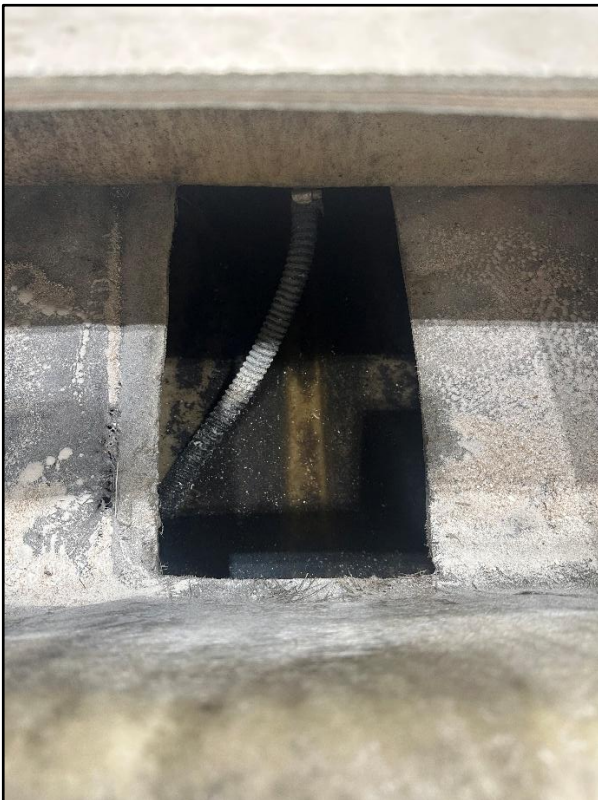
Figure 17: The drainage pipe ran from the wheelhouse and through to the hold, beneath the inner liner. Water could enter via the penetration from the hold, as the area beneath the inner liner was deeper than the floor of the hold. Photo: NSIA
