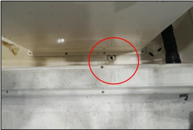
Figure 15: Drainage holes from the deck in the wheelhouse. Photo: NSIA
