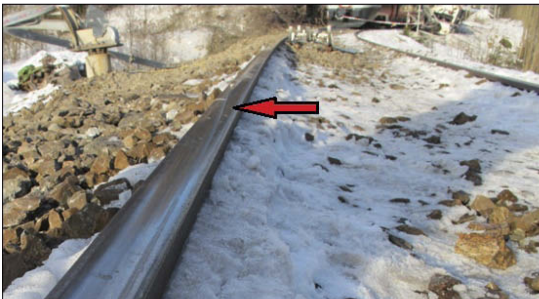
Figure 12: Derailment marks only on the left rail (photo: the AIBN).
