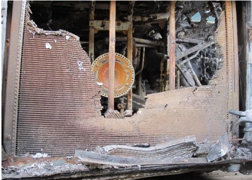
Figure 9: Radiator and fan pump (behind the round disc). Photo: AIBN
