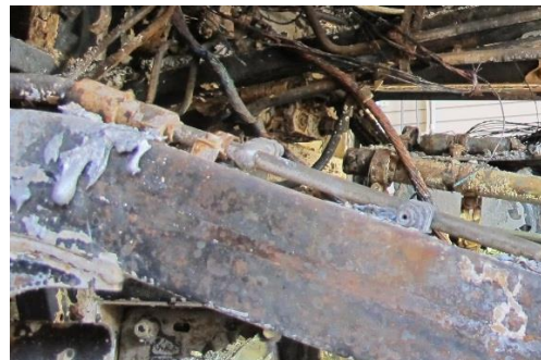
Figure 12: Nozzles from the fire extinguishing system located at the back of the engine compartment. Photo: AIBN
