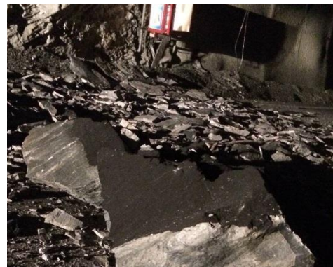
Figure 7: Close-up of fallen debris. Photo: Aurland fire service
