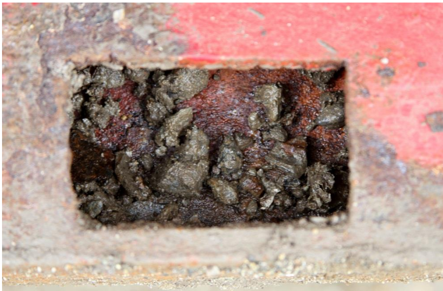
Photo 11. The hole in the fram of the hooklift container into which the securing devices fitted. Observe that the hole was filled with gravel and dirt.
