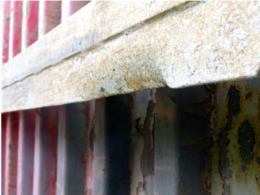
Photo 28. Damaged inner flange on the truck container.
