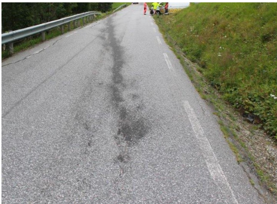
Figure 12: The road viewed forwards from the point of collision in the direction in which the coach was being driven: there is a minimal road shoulder and a steeply sloping ditch. Traces of oil leaks can be clearly seen in the photograph. Source: Norwegian Public Roads Administration
