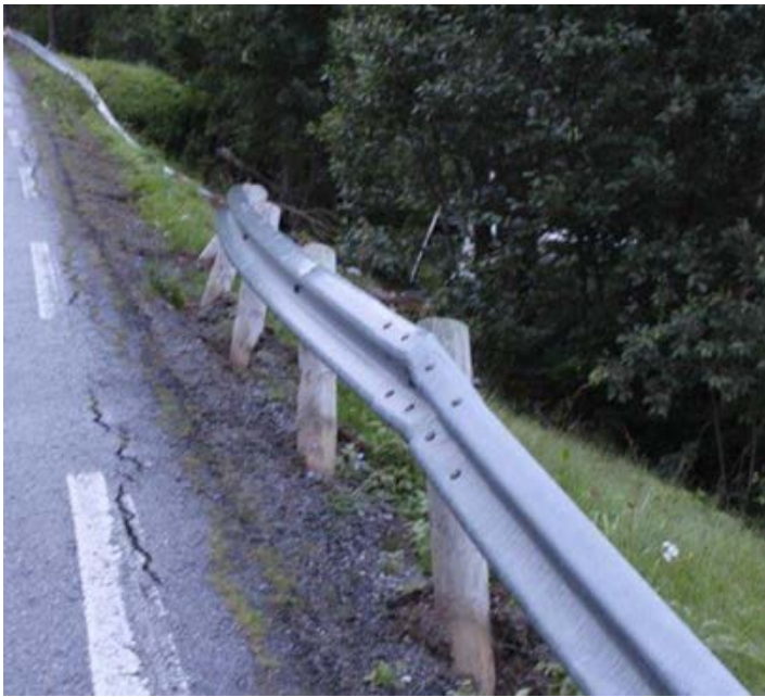
Figure 13: The crash barrier was bent down and the wooden posts loosened from their foundation when the coach rolled over. Photo: Norwegian Public Roads Administration
