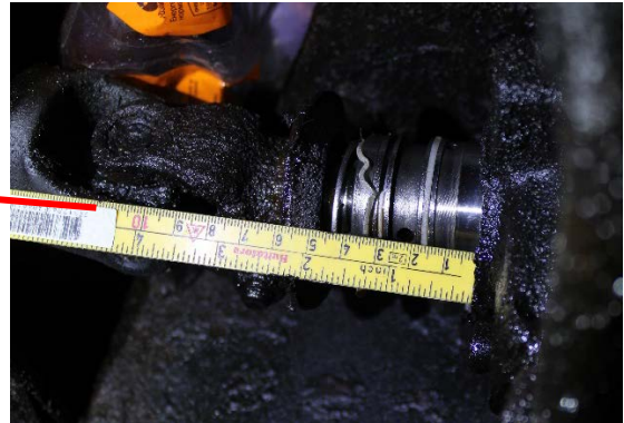
Figure 15: The fracture in the steering worm and the oil leak. The outward displacement of the axle in the steering worm was measurable. Photo: Norwegian Public Roads Administration
