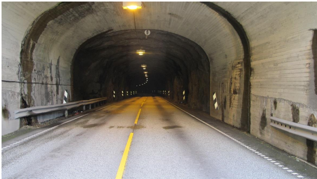
Figure 8: The photograph was taken from the tunnel opening in the direction in which the passenger car was travelling. Photo: AIBN
