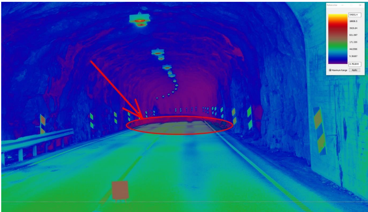
Figure 3. The image shows the threshold zone of the Raunekleiv tunnel in false colours. The false colours are assigned to pixels with certain levels of luminance. The luminance scale is shown in the top right-hand corner of the image. The red oval marks the point where the lighting is dramatically reduced.
