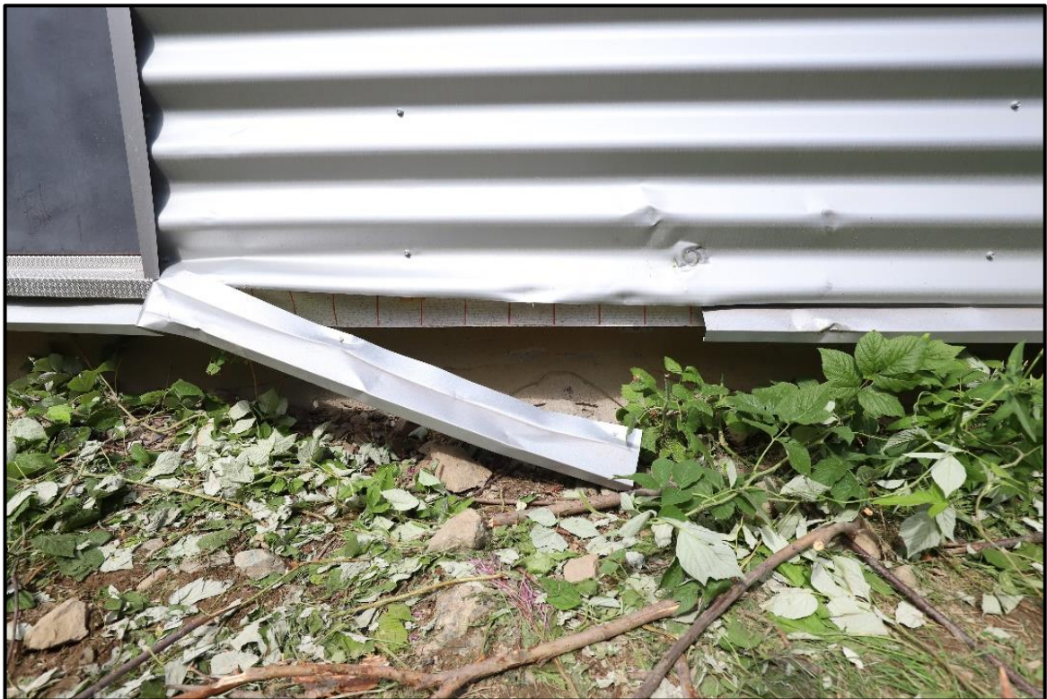
Figure 6: An aluminium strip on the wall of the industrial building was torn off in the crash. Photo: The police
