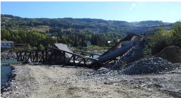
Figure 4: Temporary road by the western end of the bridge photographed on 7 September 2022. Photo: NSIA
