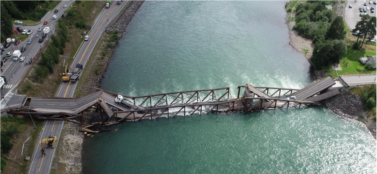
Figure 1: Tretten bridge at 14:45 on 15 August. Photo: NSIA
