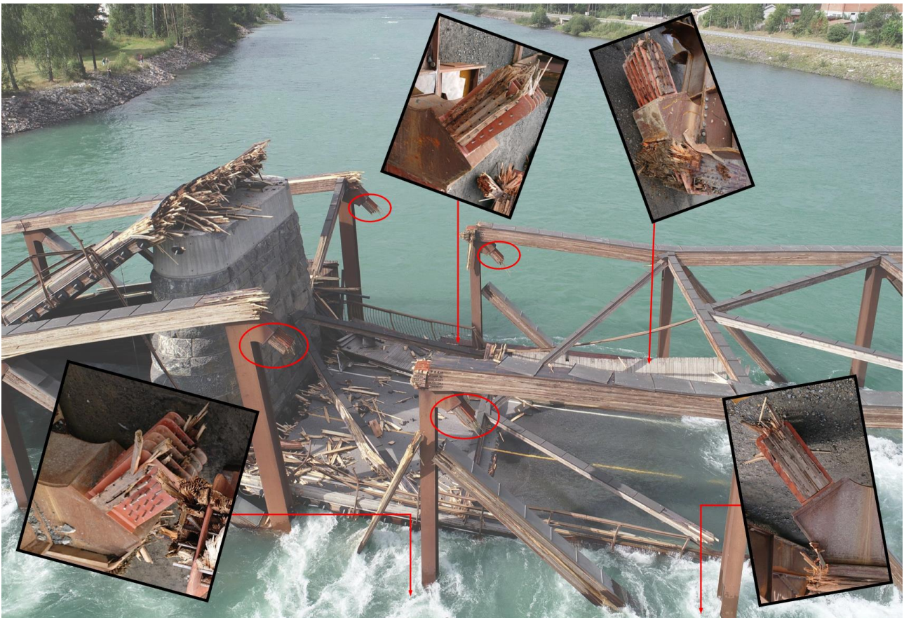
Figure 1: Red rings around the upper connections, and images of the connections that was under water, and attached to the diagonals in the main span towards the western river foundation (axis 2). Illustration: NSIA
