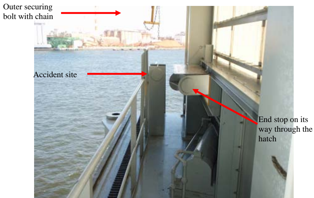
Figure 2: Accident site on top of the aft girder on starboard side, in gantry crane no. 1.
