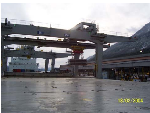
Figure 4: Open gantry crane.
