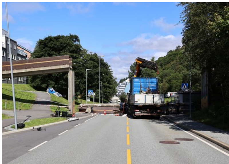
The accident site. Photo: NPRA
